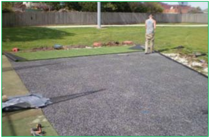
Synthetic grass being laid over shock pads and rubber safety logs installed around perimeter
